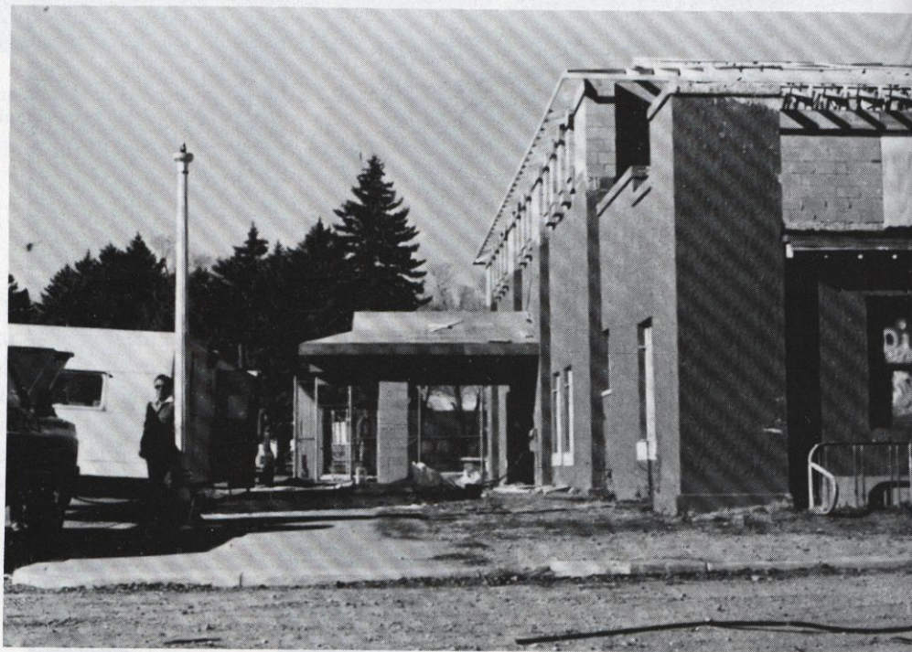
Outside the 40 year old Works Progress Administration building as Salida Hot Springs Swimming pool, is getting a new entry way, and earlier, high concrete eaves were knocked down to give a more modern appearance.
