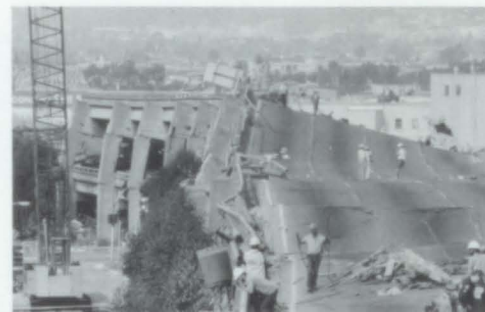
REGISTERING 6.9 on the Richter scale, a catastrophic earthquake rocked Northern California Oct. 17, killing at least 62 people, caving in bridges and freeways, igniting fires and causing widespread building damage. It hit during the evening rush hour.
