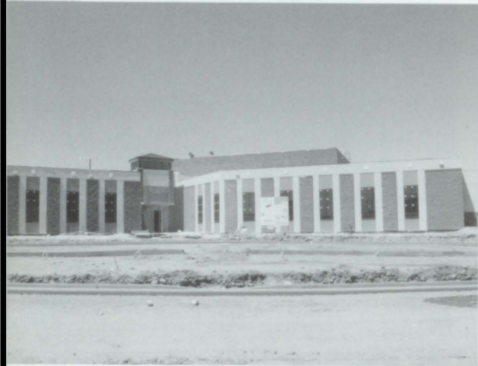
As of May, this is how the new middle school is coming along. It is 89% complete and is scheduled to open in time for next school year.
