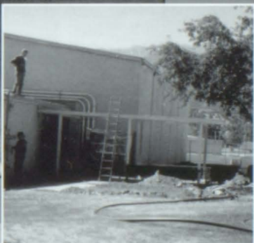
School grounds were torn up this summer for a new sprinkler system to be installed.
