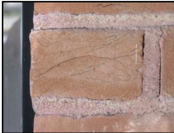
Figure 27. Dry pressed brick, end view. Cracks in brick are from hand placement of clay in the form. Brick probably laid with bottom up. Note red tinted mortar and stuck joints, vertical and horizontal.
