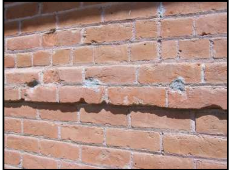
Figure 36. Spalled and patched brick.
