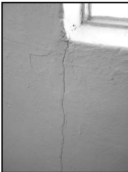
Figure 52. Vertical crack in window sill, west wall in Hall.
