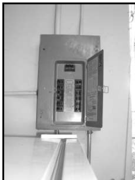
Figure 65. Main electric breaker box on north end of east wall, east end of kitchen.
