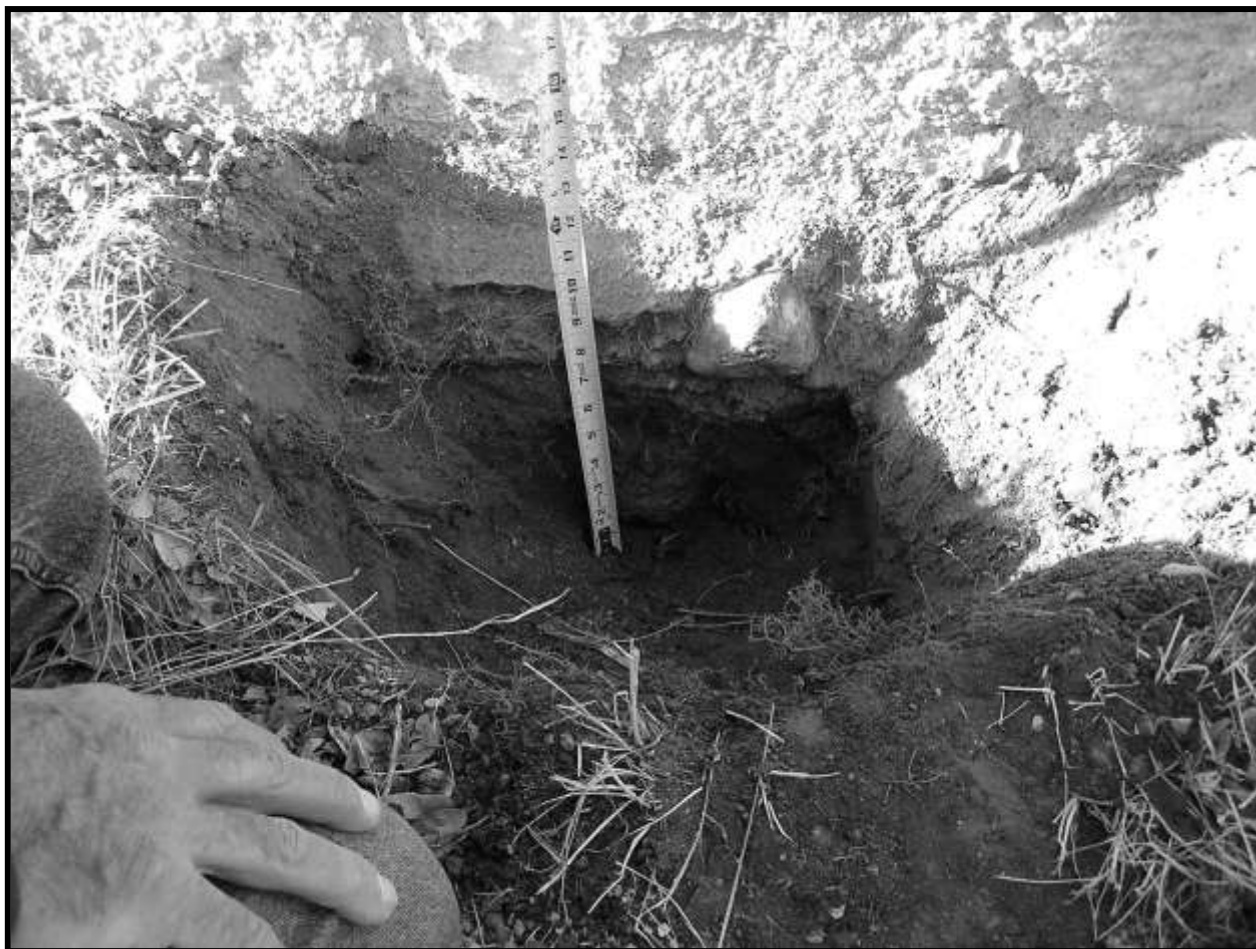
Figure 18. Stone rubble exposed below pebbledash stucco parge coat. East end of south wall, looking north.
