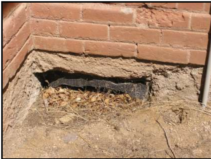
Figure 1. Crawl space vent, west wall at intersection of entry Wall. Note more spalled and poorly patched brick.
