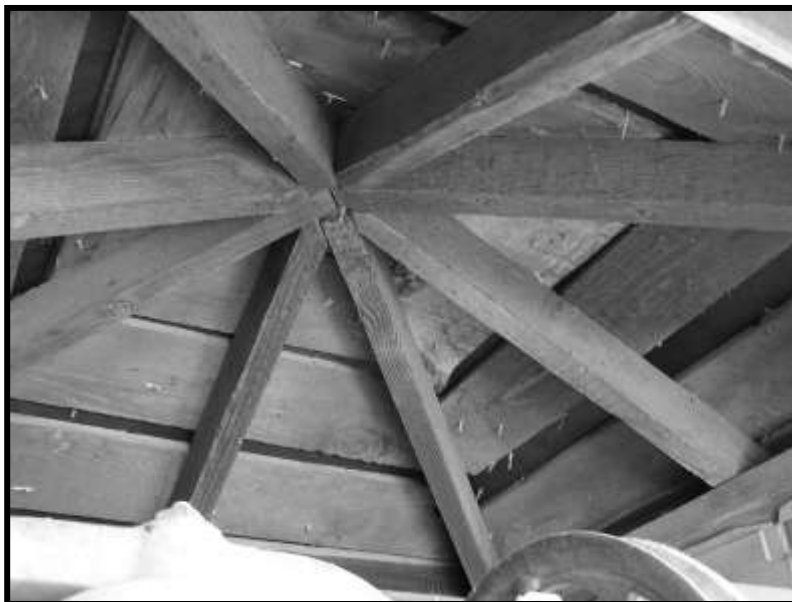
Figure 20. Belfry roof framing. All eight rafters extend beyond belfry sidewalls to form overhang.
