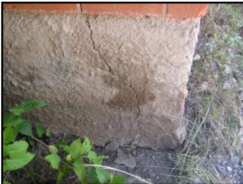
Figure 17. Foundation crack, east wall at northeast corner. Crack continues up to end of window sill (See Figure 52 for same crack on interior). Stain on pargeting is probably due to moisture entering the crack.
