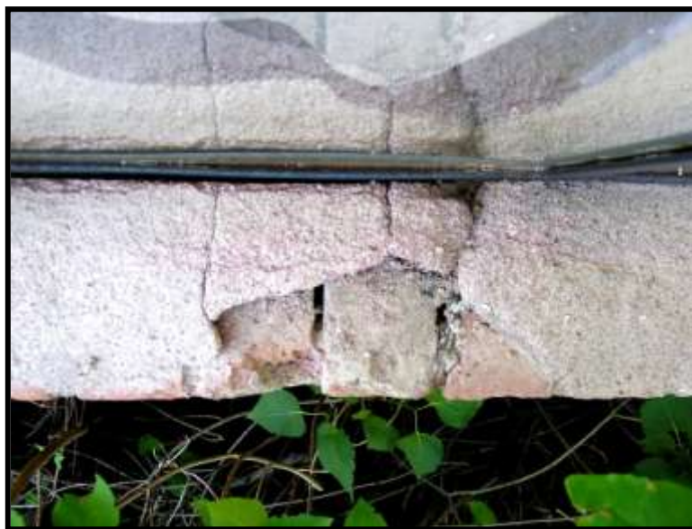
Figure 34. Mortar wash, east wall northernmost window. Deterioration is typical of similar in several locations.
