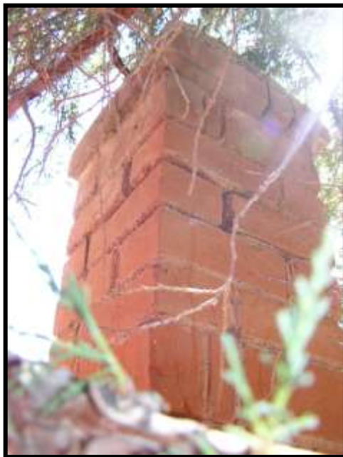
Figure 32. Northernmost entry pilaster, looking southwest from behind. Note open mortar joints.
