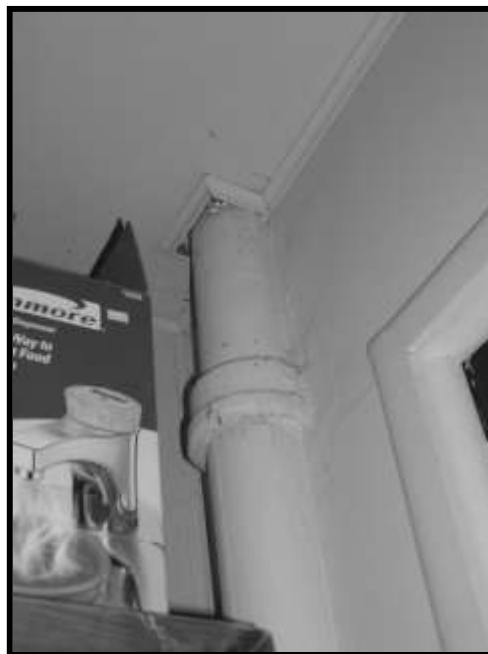
Figure 63. Cast iron waste vent in Storage Room (former restroom.)
