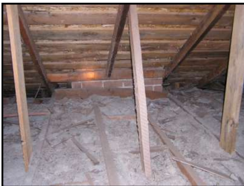
Figure 19. Main roof framing in attic, looking west. Note ceiling. Framing spacing different than roof and chimney at eave.
