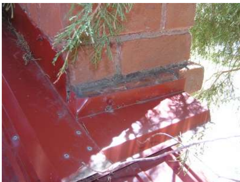
Figure 38. Roof flashing around brick pilaster, north side of entry. Note crude fit and non-integrated work. Interfaces depend on sealants to keep water out.
