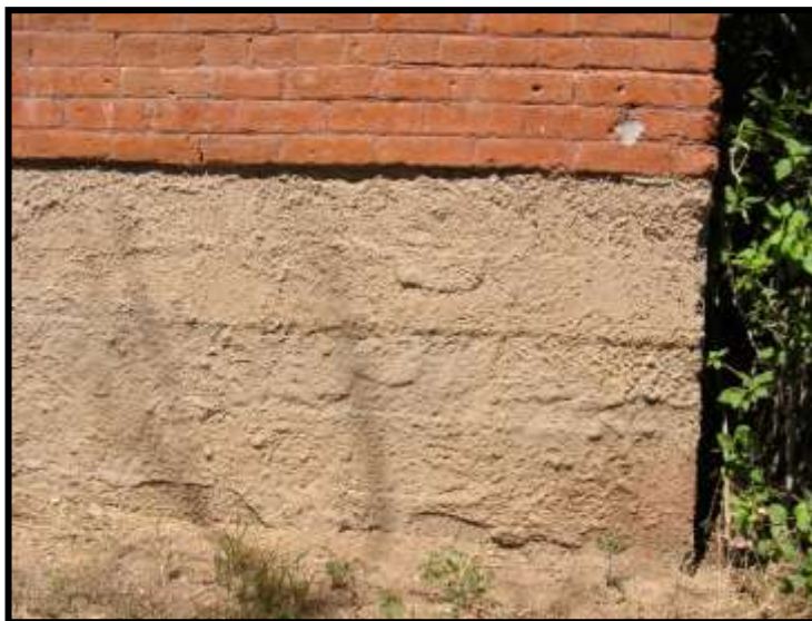
Figure 12. Foundation wall. South wall, southeast corner, showing parget coat over horizontal formboard marks.
