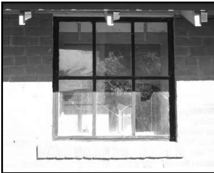
Figure 46. Restroom window, west façade. Entire window is operable as a pivoted sash.
