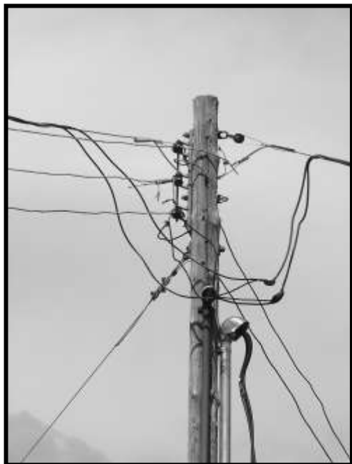
Figure 66. Power pole off the northeast corner of the building. The three lines to the left are the current service lines to the building.
