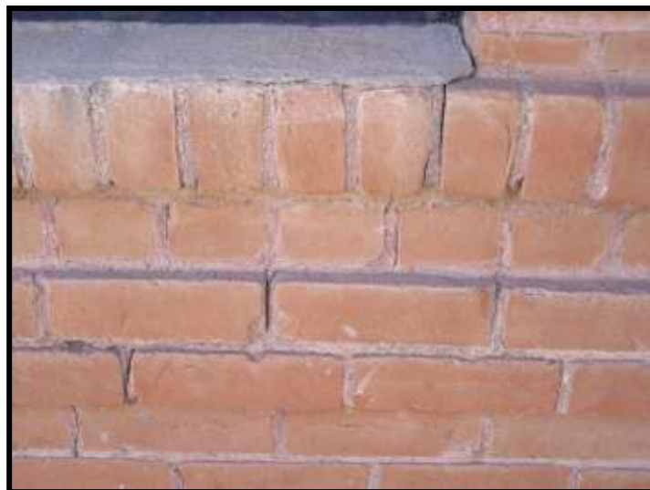
Figure 30. Crack at sill and below, south end of sill, northernmost window in Hall.
