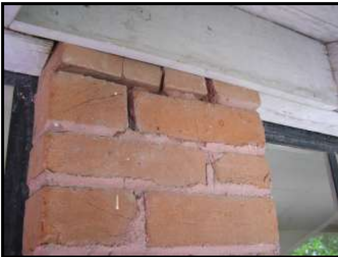
Figure 37 (Left) Brick pilaster between windows, south portion of west wall. Note red tinted mortar with struck joints, spalled brick corner, and open joints at upper courses.
