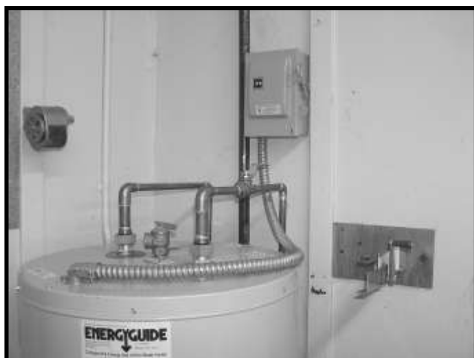
Figure 64. Electric water heater with switch at wall. Located in west end of Kitchen.
