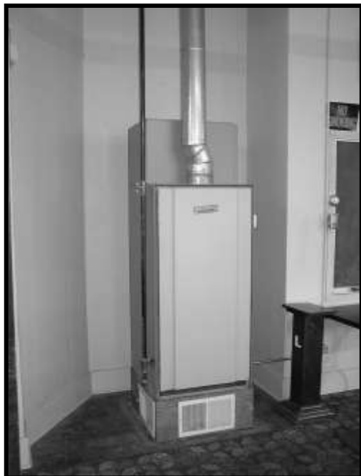
Figure 60. Propane fired forced air heater in niche in North Classroom.
