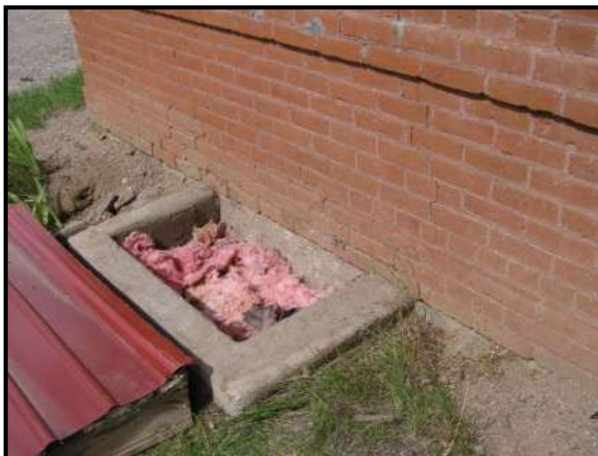
Figure 14. Crawl space entry, north end of west wall. Below the pieces of fiberglass batts is more insulation of various types.
