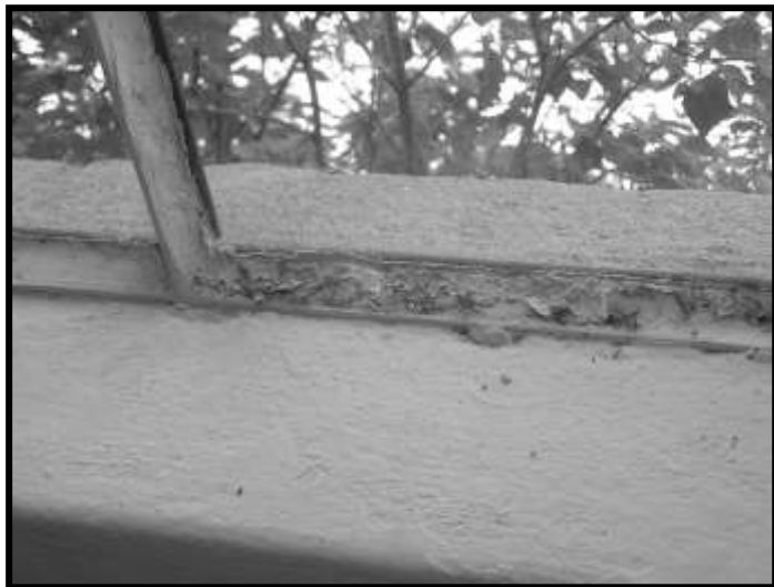
Figure 44. Window putty, east wall. Poor condition.
