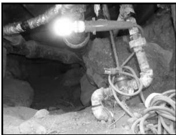
Figure 62. Plumbing in crawl space, near crawl space entry.
