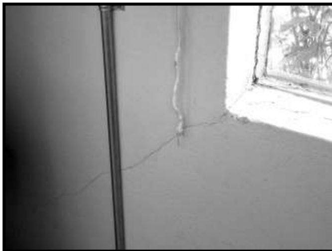
Figure 50. Diagonal crack from sill down to left in North Classroom. North end of sill, north window, east wall. (See Figure 17 for same crack on exterior.)
