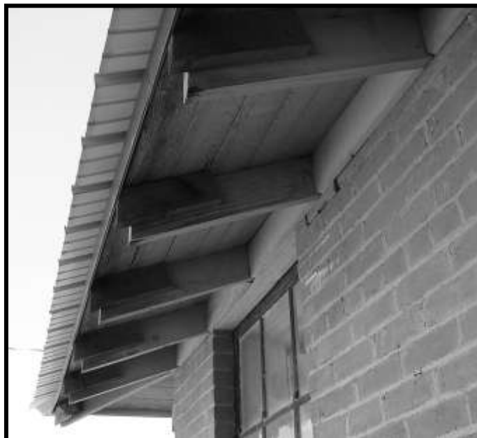
Figure 24. Roof overhang at north end of west façade, looking northerly. Notice scabbed-on 2x4s and excess roofing overhang.
