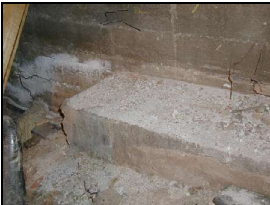
Figure 18. Foundation and stepped footing, west wall, basement. Note efflorescence.
