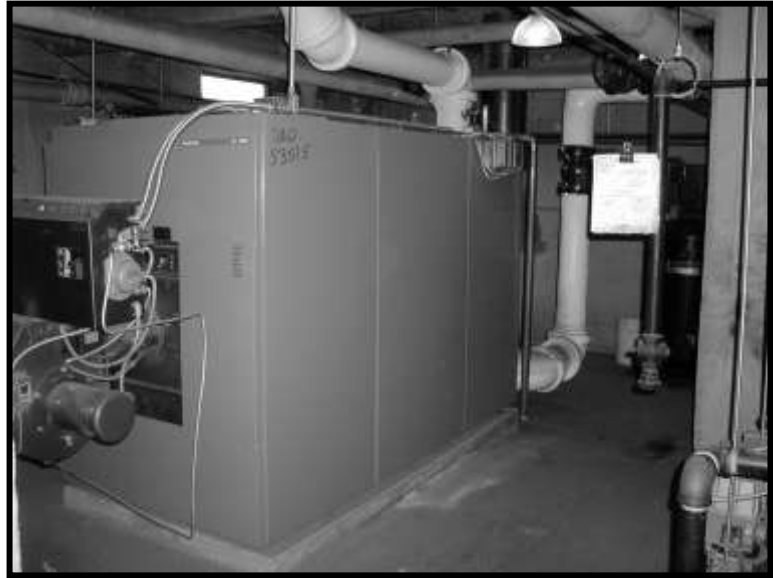
Figure 82. One of two new boilers
