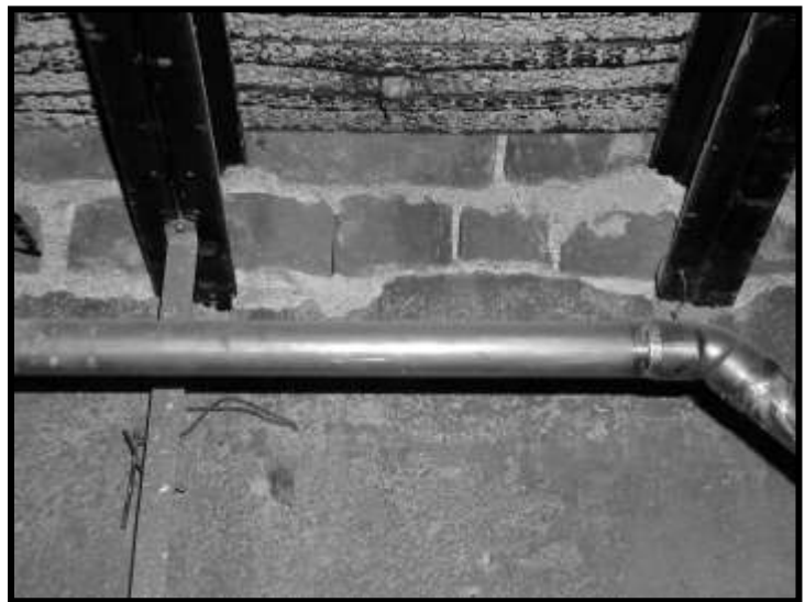
Figure 22. Double steel channel joists bearing on exterior foundation wall. Note brick infill between joists. Brick is the water table backing
