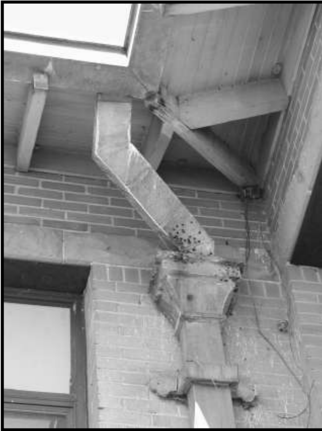
Figure 52. Downspout, south end of pavilion projection, east wall. Note bullet holes in leader and conductor head, and water stained rafter tail ends.
