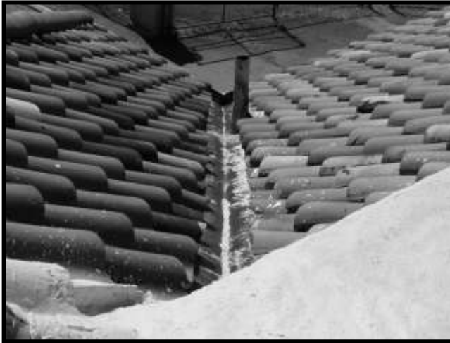
Figure 48. Southeast roof valley flashing. Note waste vent through the flashing.
