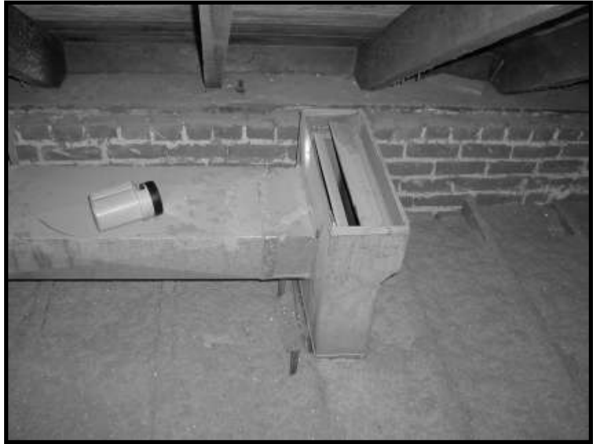
Figure 83. Ventilation duct in attic with damper.
