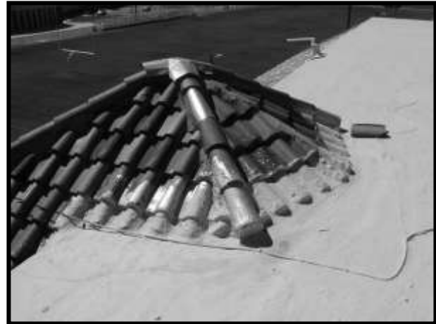
Figure 45. Makeshift metal flashing at top of point of the east pavilion projection roof.
