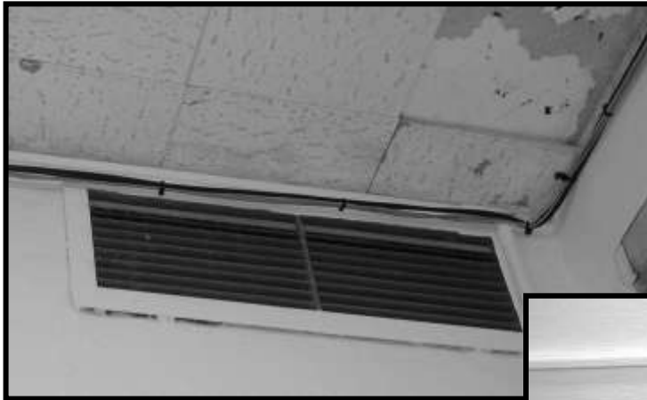
Figure 75. Ceiling at northeast corner of Room 117. Note missing tile, and stains on those at the edge of the ceiling. Also note exposed wires and wire mold running around the top of the wall.
