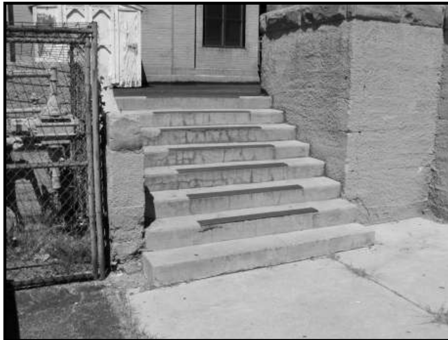
Figure 38. Concrete stair to boiler room roof. Note poor condition and handrail to left with no coping.
