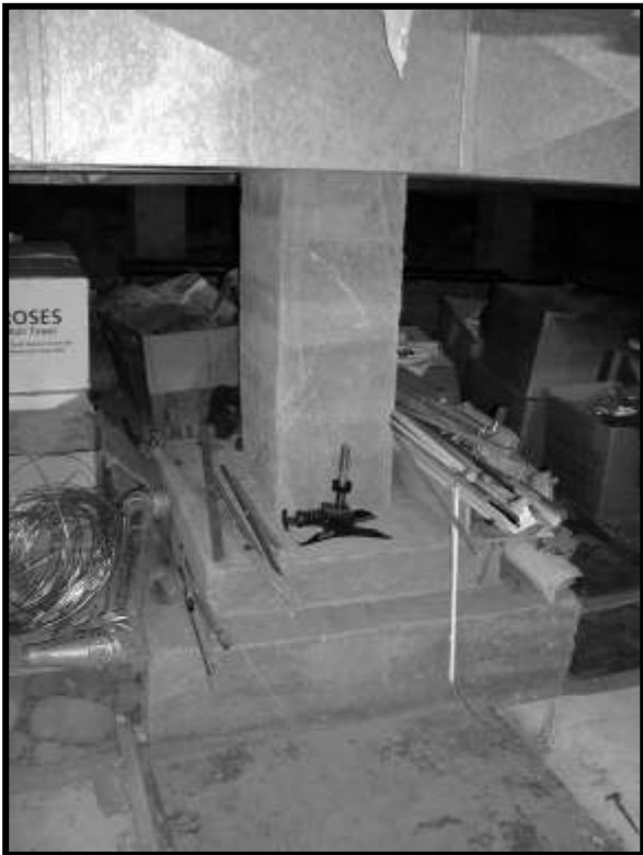
Figure 21. Interior concrete column (pier) with footings. Note lack of efflorescence. Ventilation trunk duct overhead.
