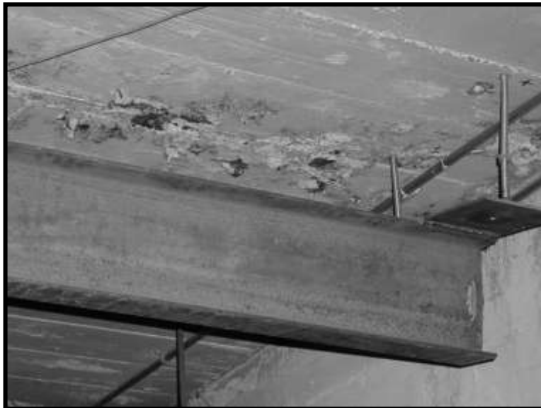
Figure 47. Boiler room concrete slab ceiling. Note flaking paint on ceiling above steel beam.
