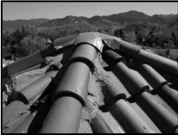
Figure 46. Interface of tile roof and semi-flat roof. Note roof coating mopped up over tiles and sheet metal cap also seen in Figure XX
