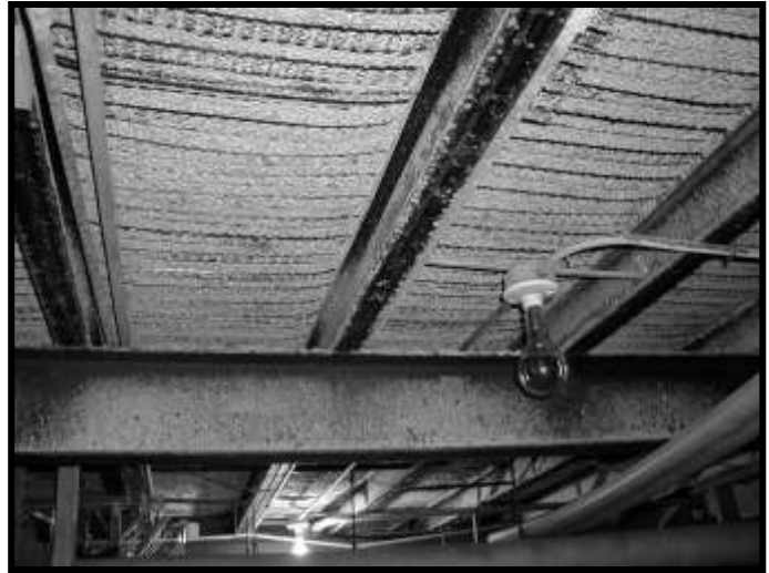
Figure 20. Underside of first floor showing concrete oozing through diamond mesh rib lath supported on double 6" steel channels on I beam (background).
