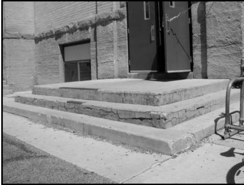
Figure 37. Concrete stoop at south entry doors. Note cracking and crazing, especially at top risers.
