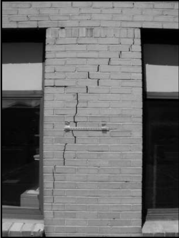
Figure 35. East wall, between third and fourth windows from south. Large continuous crack. Note broken bricks.
