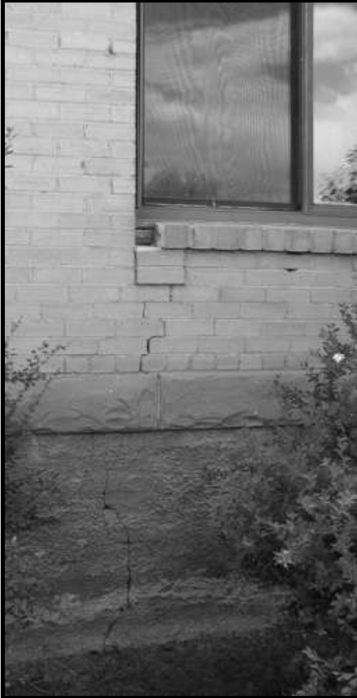
Figure 33. East wall, second window from south. Diagonal cracking under window. Note pebbledash stucco coat on foundation wall beneath sandstone water table to grade
