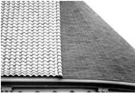
Asphalt shingles are an incompatible replacement substitute for the original Spanish clay tiles. Photo: NPS files.
