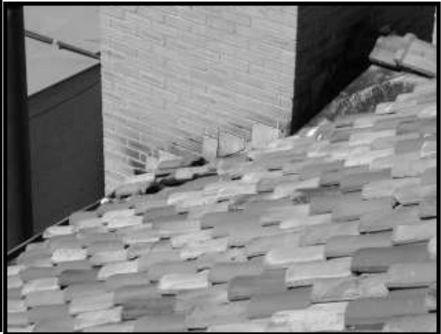
Figure 49. Stepped flashing and saddle flashing at chimney-roof interface.
