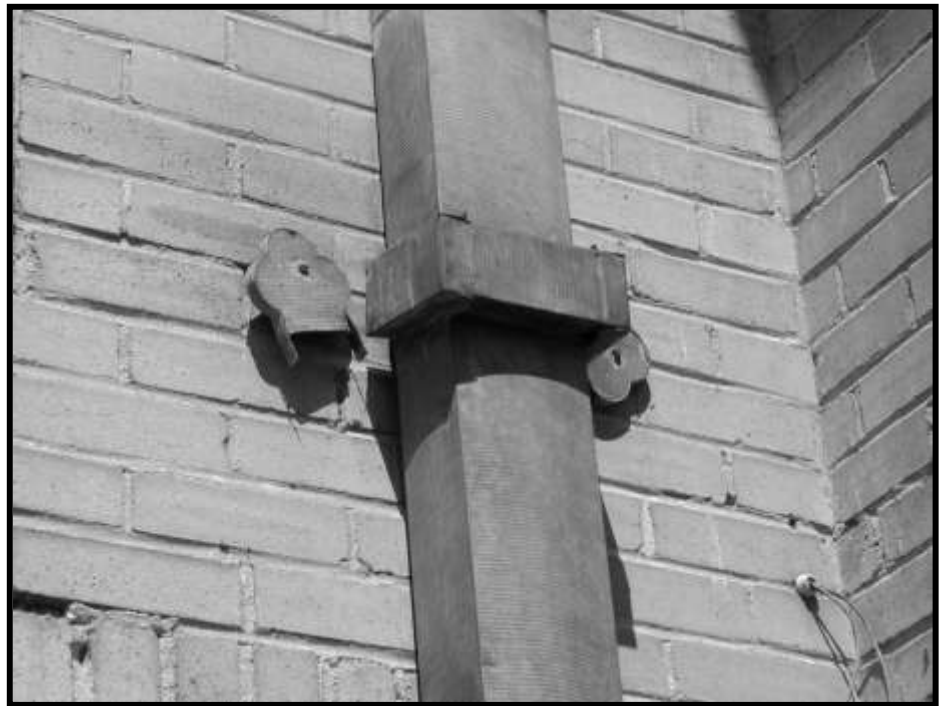
Figure 53. Broken downspout wall anchor bracket.
