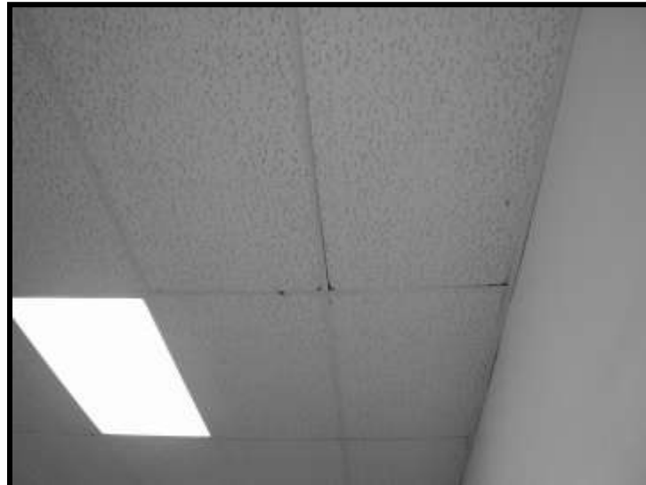
Figure 79. T-grid lay-in ceiling panels in main floor corridor.
