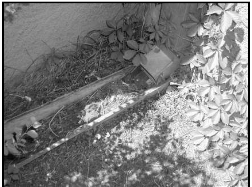
Figure 51. Downspout at south end of east wall. Discharge is into sheet metal trough that is sloped backward against building.
