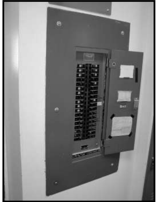
Figure 85. Sub-panel in first floor hall, Kesner Building.
