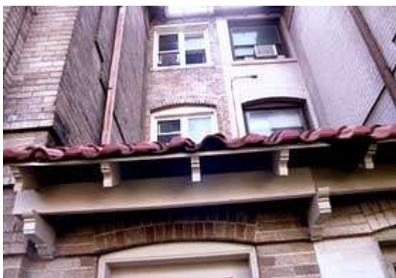
An eave closure or birdstop to keep out birds is notably absent from the replacement tile in the center of the bottom row. Photo: NPS files.
