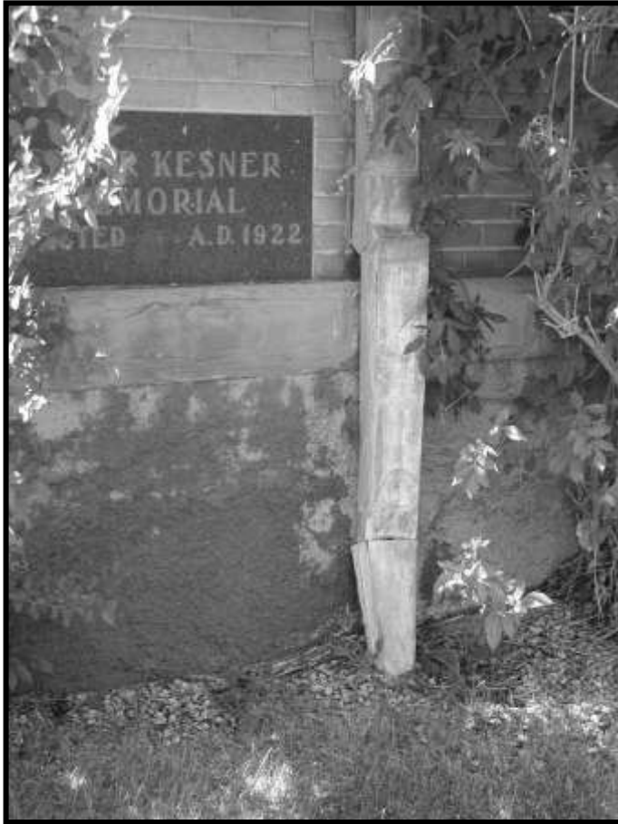
Figure 50. Downspout at east end of north wall. Discharge is into metal pipe in ground.
