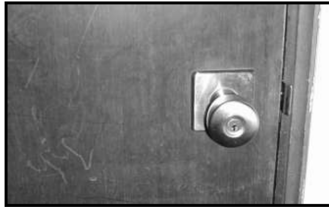
Figure 64. Exterior (hall side) door knob. Note scratched condition of door.
