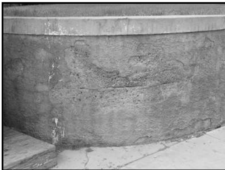
Figure 9. Concrete retaining wall curved corner with concrete cap and pebbledash stucco finish below. Note horizontal line in concrete showing two concrete pours.
