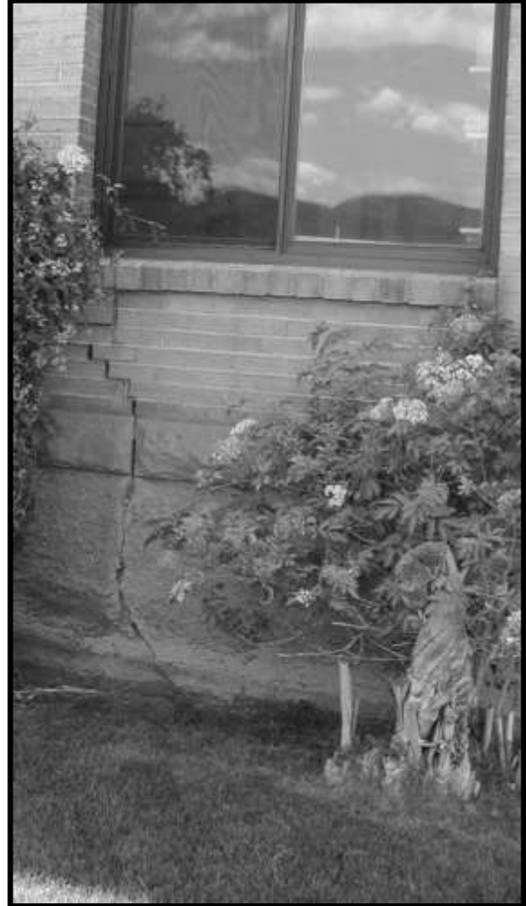
Figure 32. East wall, third window from south. Diagonal cracking under window.
