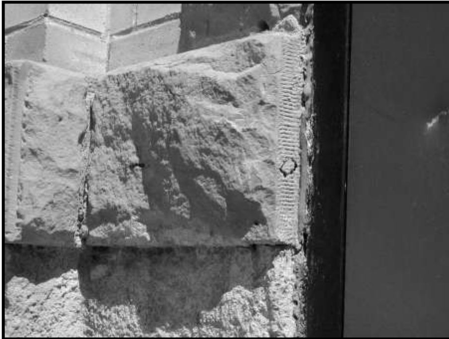
Figure 27. Sandstone water table (inside corner) showing pebbledash stucco below, brick above, door jamb at right.
