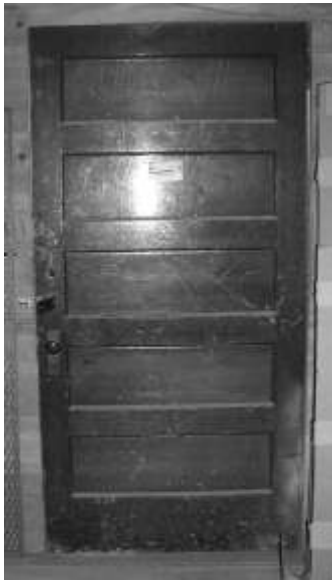
Figure 62. One of three historic five-panel doors in the basement. Bottomrail has been cut down to fit new opening.
