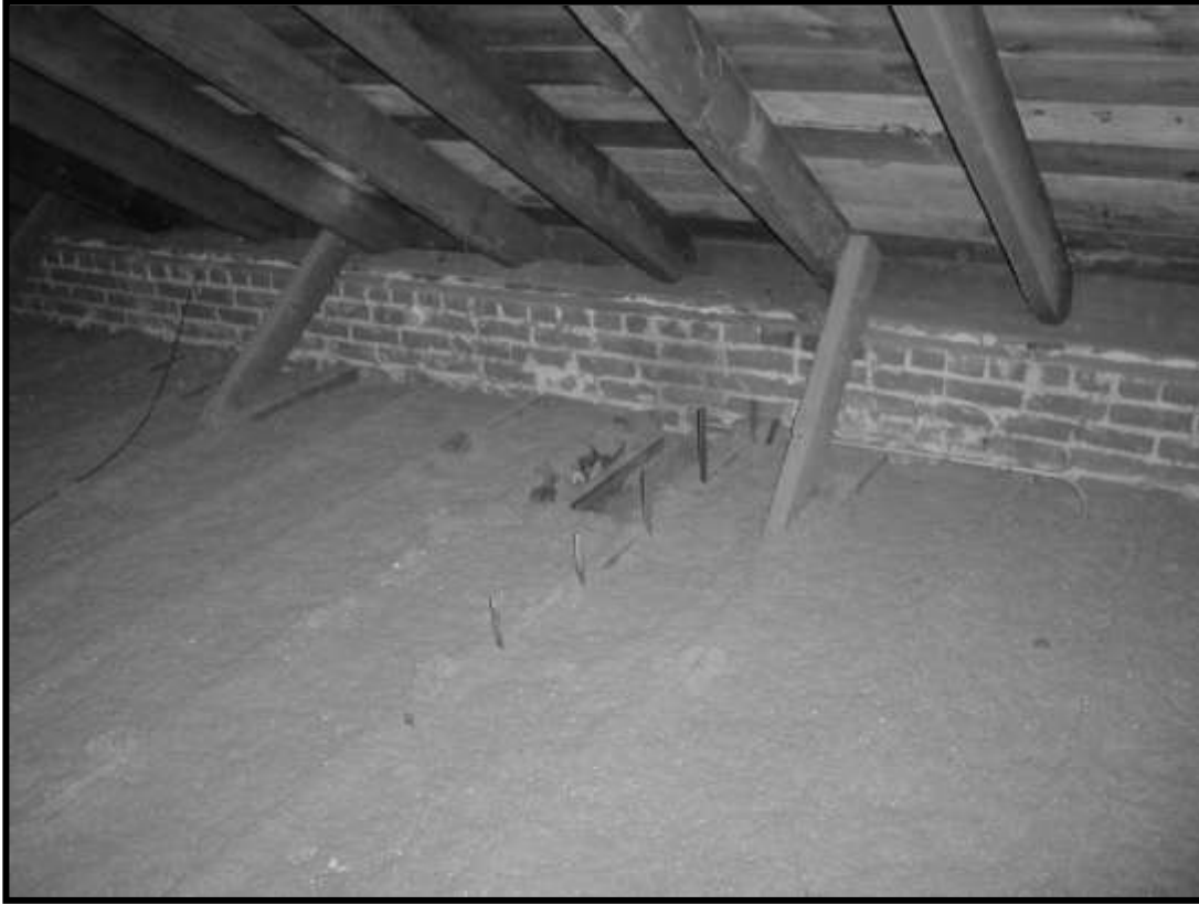
Figure 25. Blown-in insulation in attic with steel wall framing channels protruding through ceiling.
