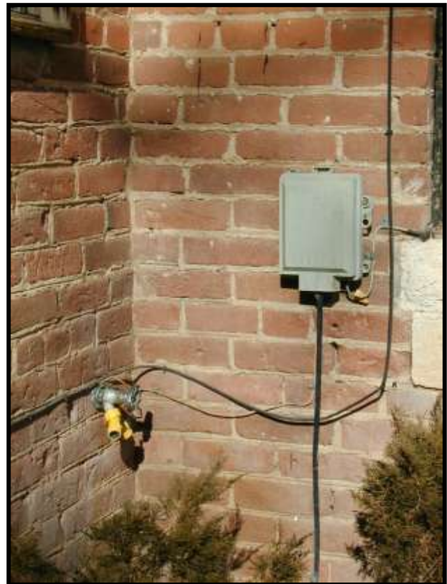
Figure 11. Looking northwest at corner of east Entry wall and South Main Building wall, across planting bed. Note wide area of lighter color brick and eroded brick beneath faucet.
