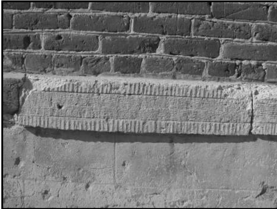
Figure 24. Watertable in fair condition. Note scored stucco parget coat below. This piece of watertable near the south end of the east well, main building, is a good candidate for use as a pattern for new watertable pieces.
