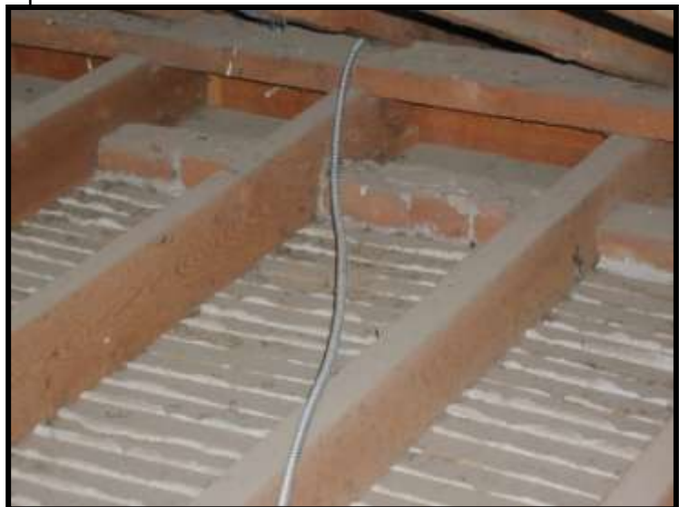
Figure 12. Roof and ceiling framing at exterior wall plate. Note bricks between ceiling joists.
