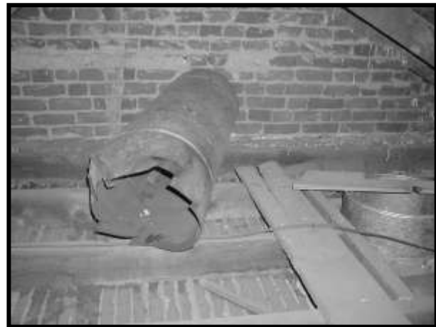
Figure 21. Loose pipe on ceiling at northwest corner of building.
