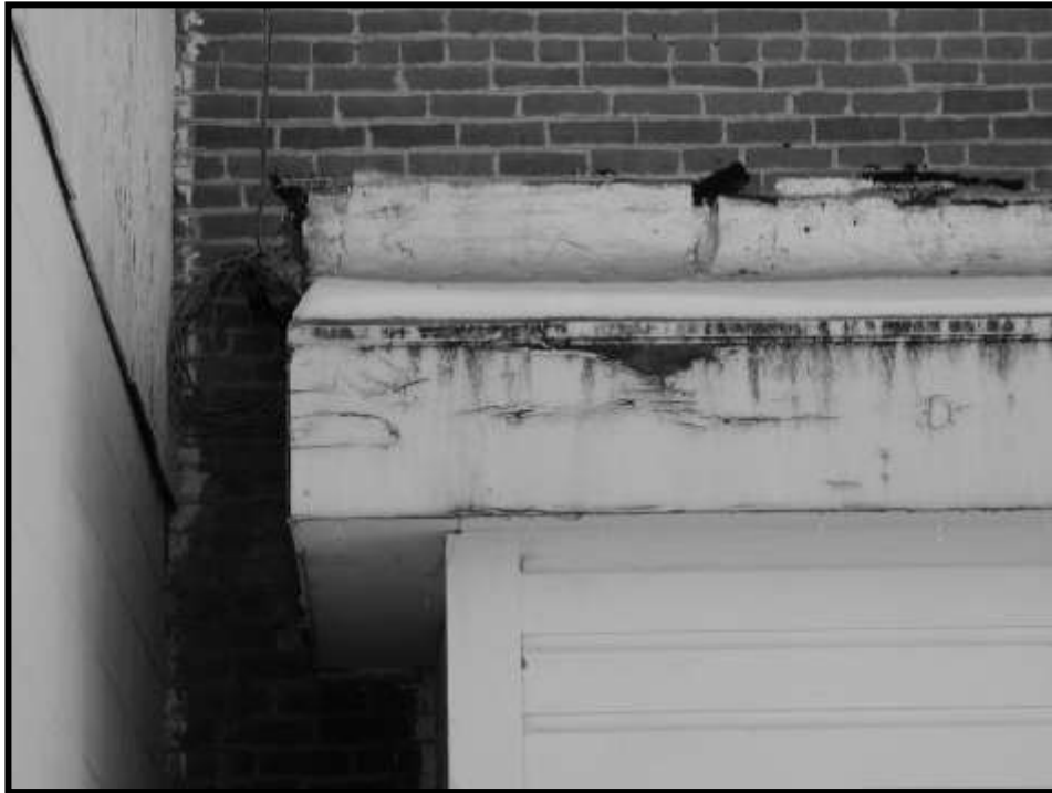
Figure 33. Storage Room, fascia and flashing. Northeast corner of Storage Room, looking south.
