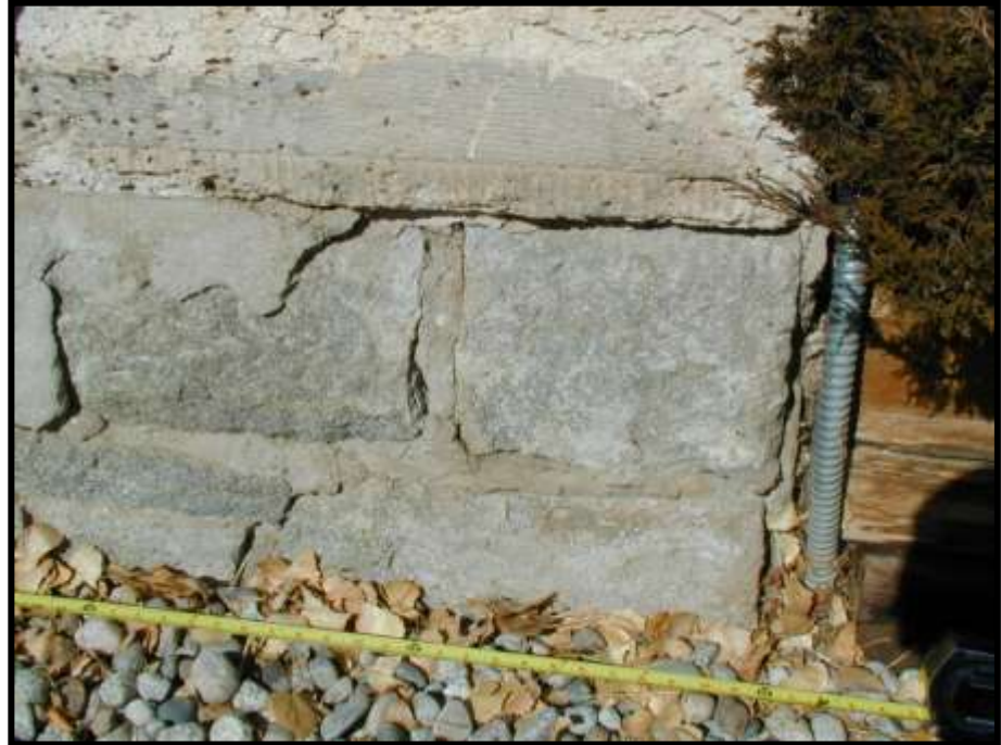
Figure 10. Foundation. Note loose parget coat at left, and deteriorating stone water table above foundation.
