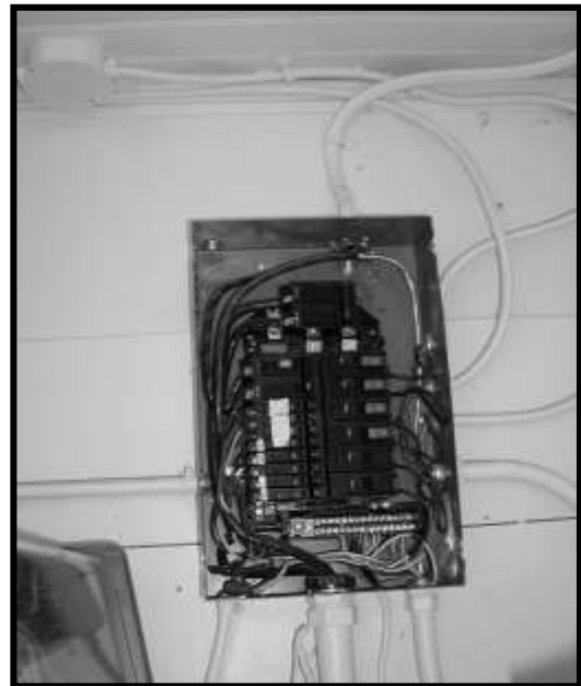
Figure 50. Electrical box in East Stair. Looking east.
