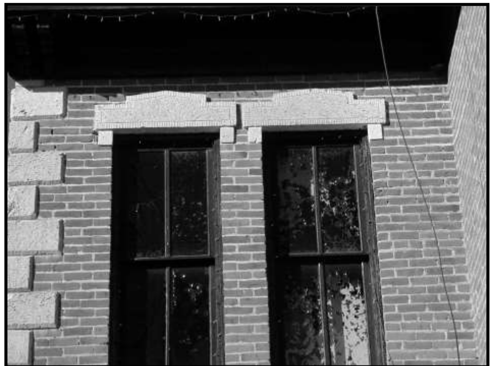
Figure 23. West pair of windows on south façade. Both window heads are in good condition.
