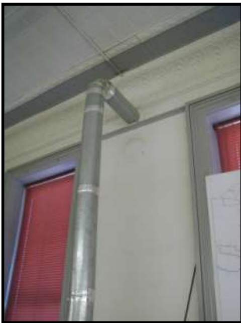
Figure 29. Stovepipe in Town Hall. Note former stovepipe hole below picture rail, plastered up. Looking northeast.
