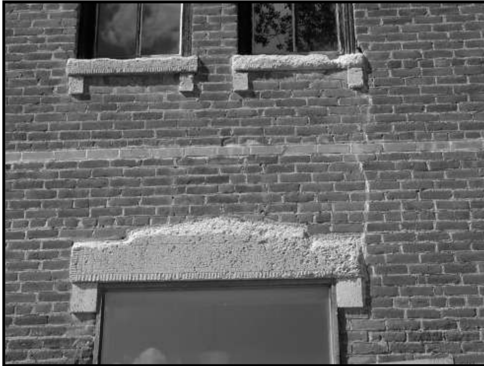
Figure 22. South façade, looking north. Decorative head at entry door, in poor condition. Left window sill above in fair condition. Right window sill above in poor condition.
