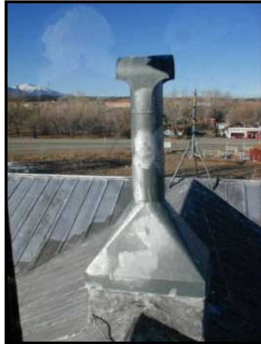
Figure 26. Center chimney above roof looking north from Cupola. Note silver paint on brick and cracked roofing cement.
