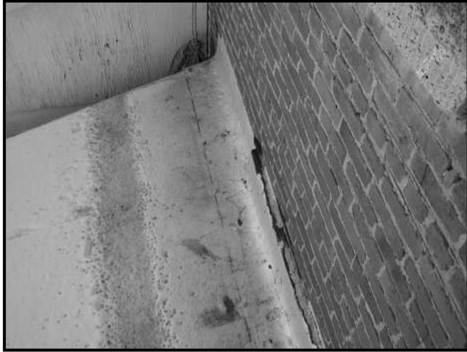
Figure 34. Storage Room flashing and roof from exterior fire stair. Southeast corner of Storage Room, looking east.
