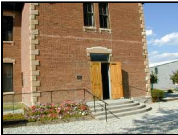
Figure 15. Note lighter colored brick course at tie rod above entry door. Looking northeast.
