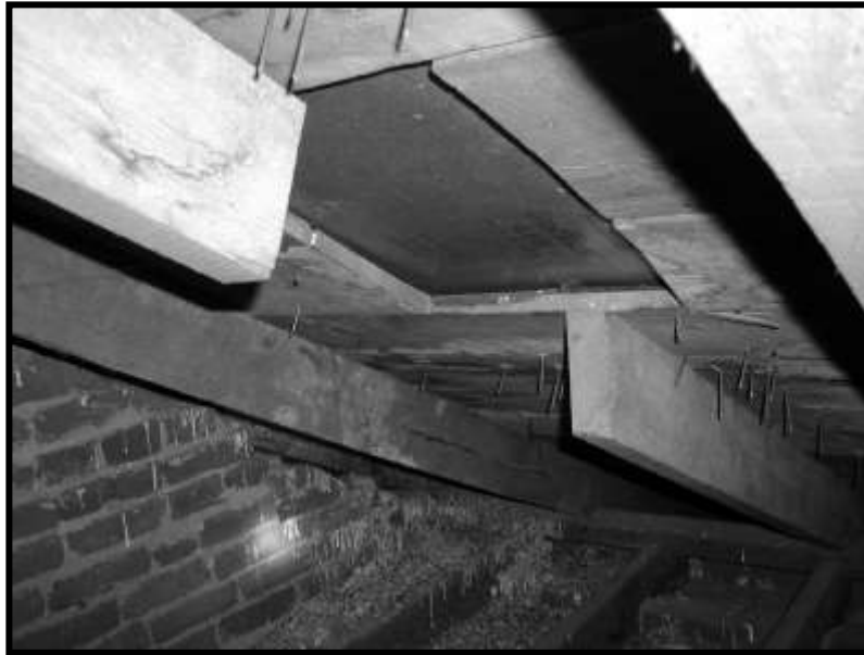
Figure 22. Roof rafter sawn through at location of 15" pipe penetration.
