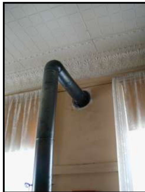
Figure 28. Stovepipe in Museum. Note stovepipe hole location below picture rail. Looking west.
