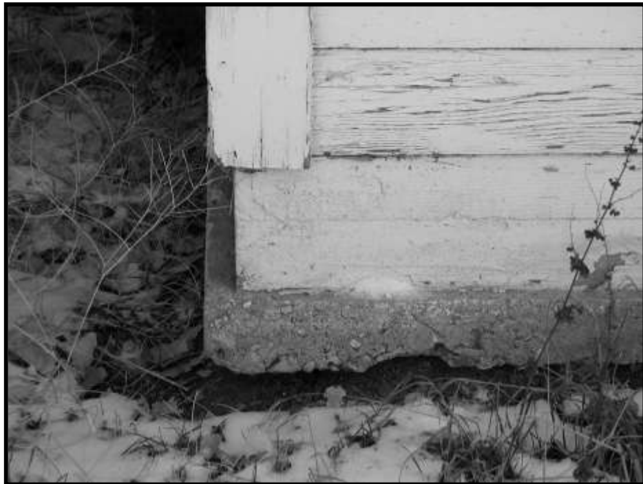
Figure 35. Storage Room slab erosion, northeast corner, looking south.
