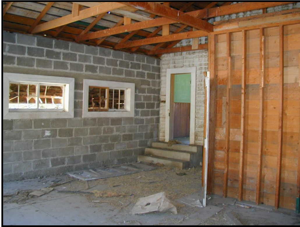
Figure 29. WPA addition, looking southeast. Note concrete steps to schoolroom door. Enclosure to right is divided into two sections, and is said to have been used for coal storage.
