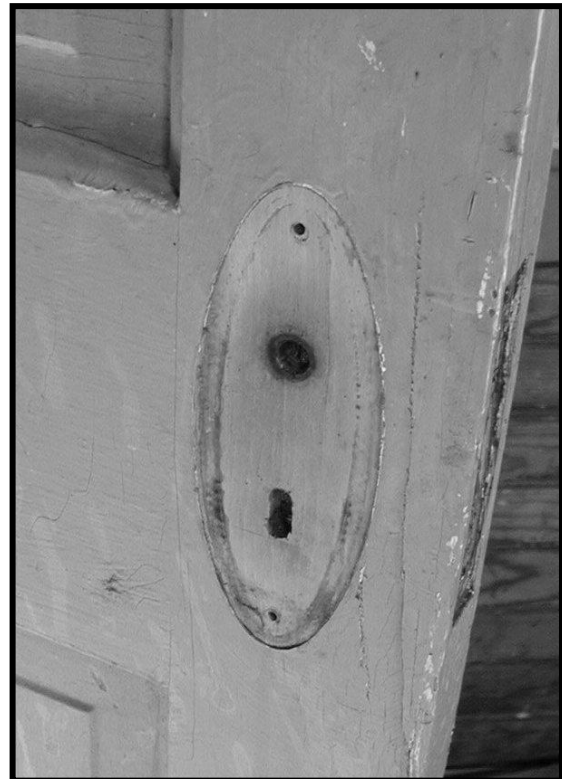
Figure 17. Ghost of knob plate on schoolroom side of door from vestibule to schoolroom. Looking east.
