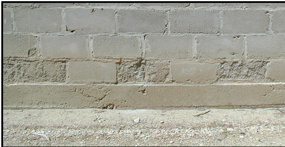
Figure 11. Concrete blocks on WPA addition, showing spalling on first course. Looking west.
