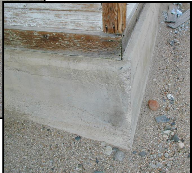
Figure 7 (left). Foundation with pebbledash stucco. Note scoring to imitate ashlar laid stone. Looking northeast.
