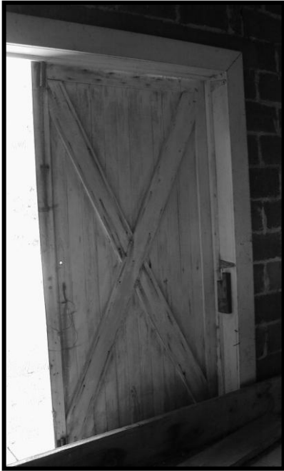
Figure 18. East leaf of vehicle door on north wall of WPA addition. Looking northeast.
