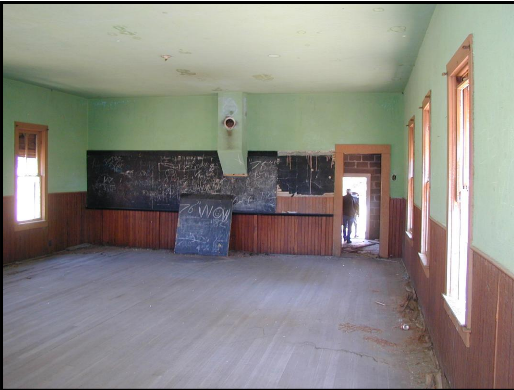
Figure 25. Schoolroom, looking north. Note rear door leading to WPA addition at right, and chimney in center. Also note blackboard.
