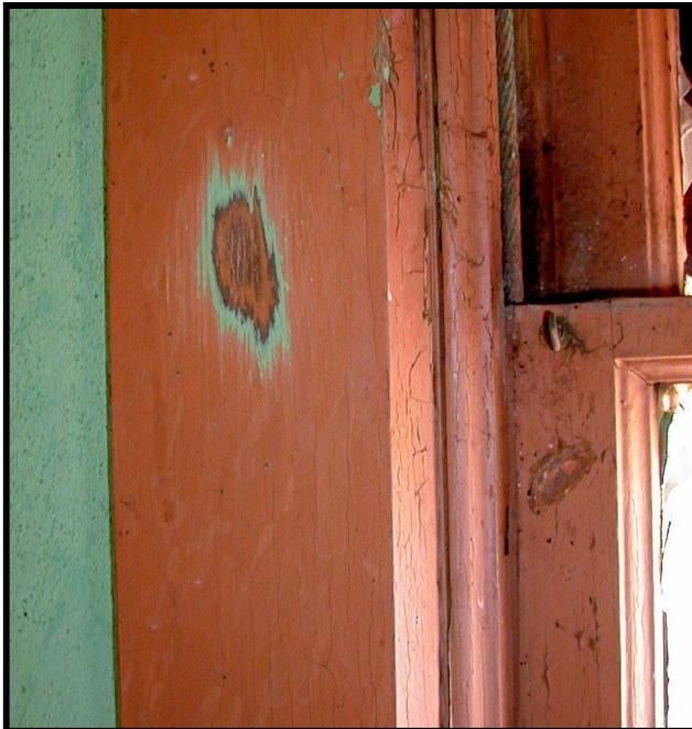
Figure 23 (left). Color crater on window trim, classroom. Note beige, green same as wall color, and grey (primer?) over wood. Note beveled trim and shaped stop molding. See hook on upper left of lower sash. This is the south window on the west wall. Looking northeast.
